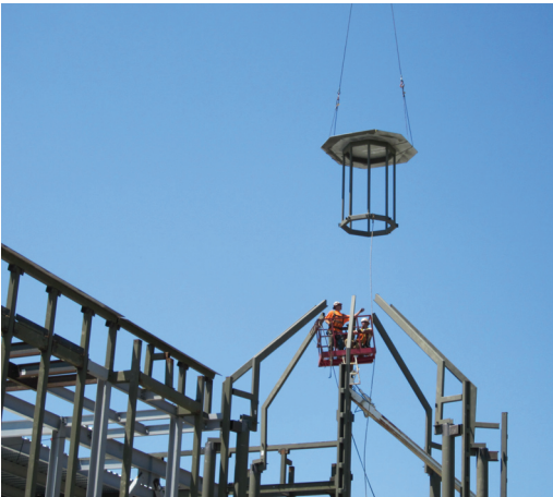
Steel Frame of New Science, Mathematics, Library Center at St. Sebastian's School
