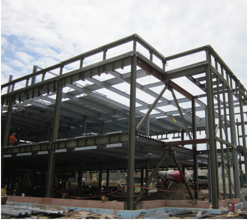
Steel Frame of New Science, Mathematics, Library Center at St. Sebastian's School
