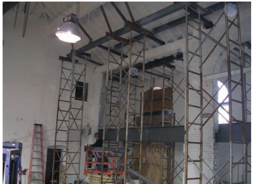
Through careful preplanning at St. Mark's School's in Southborough, Massachusetts the shoring of the existing roof structure in the Boiler Plant was recommended. New structural steel support was installed to allow for old arch brickwork to be removed.
